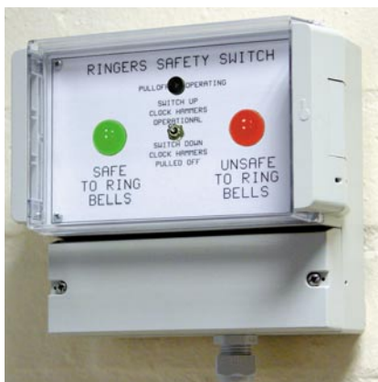
Ringing room safety switch.
