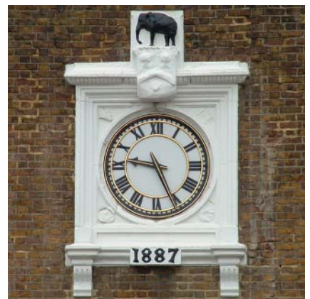
GRP replacement for a corroded cast iron dial, installed in the original surround.
