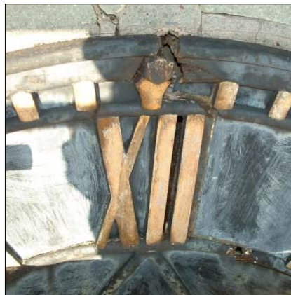
Corroded fixing which has expanded and broken the cast iron dial and stone surround.
