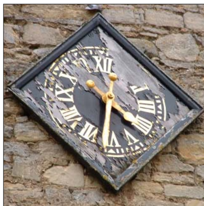
Before: wood dial deteriorated beyond repair.
