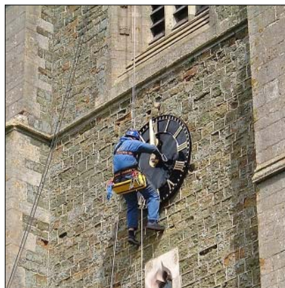
Access to a church clock dial: fully trained engineer using our safety approved equipment.
